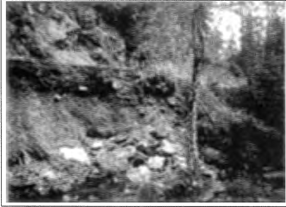
Road failures, such as this one in the South Umpqua, are significant sources of sediment. Sediment issues, whether from roads or other sources, should be considered before instream restoration projects are begun.
