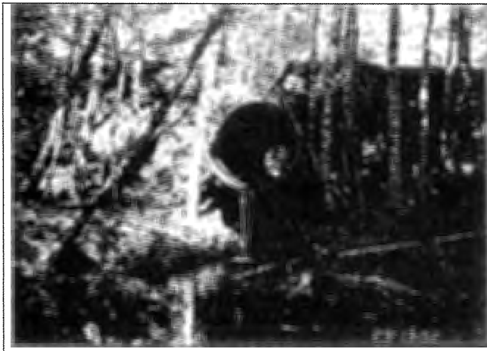
This culvert on Wolf Creek is a likely barrier to upstream migration of salmonids. If suitable habitat exists upstream, culverts such as this should be a restoration priority.
